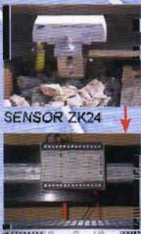
SENSOR ZK24 EVALUATION SUBSYSTEM ITR245/UTR245 INSIDE CABINET
