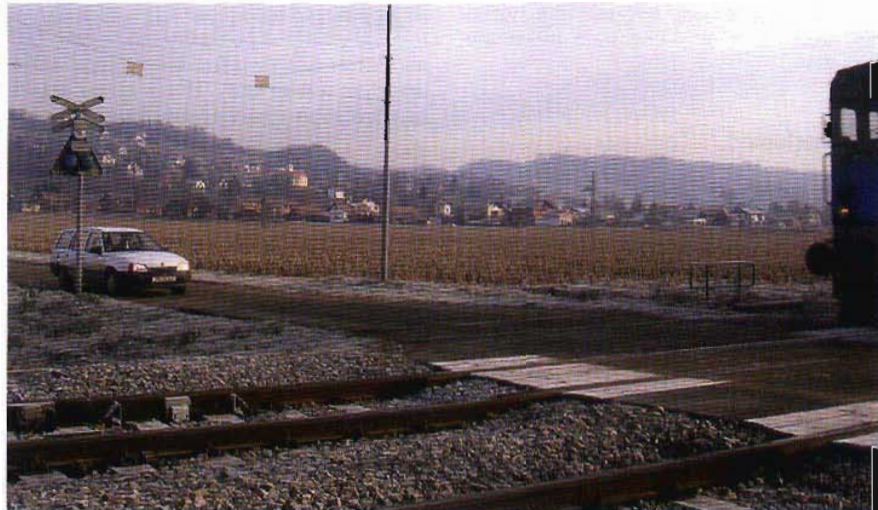
Figure 4: Wheel sensor ZK24-2 replaces old magnetic detector (not yet removed on the left) on relay level crossing
